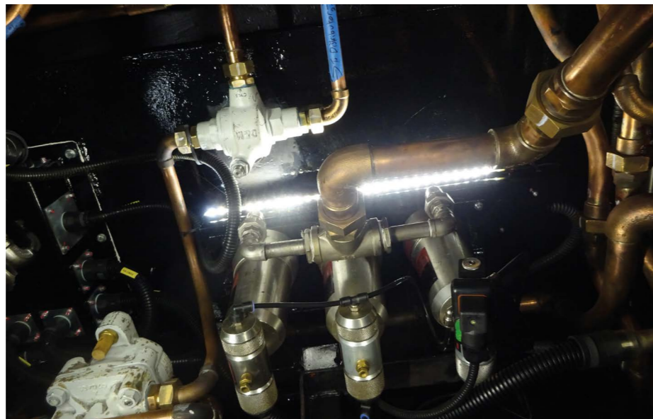
Right: New lighting strip under the front of the tender, with the air system strainer below.
