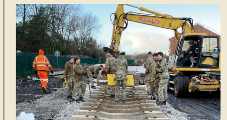
The Army moves in again. Troops of 32 Regiment making a significant contribution to the laying of track at DLW2.
