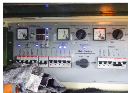
First test of the new ADA, supplying 34A, operating the two chargers and supplying the Load Bank.
