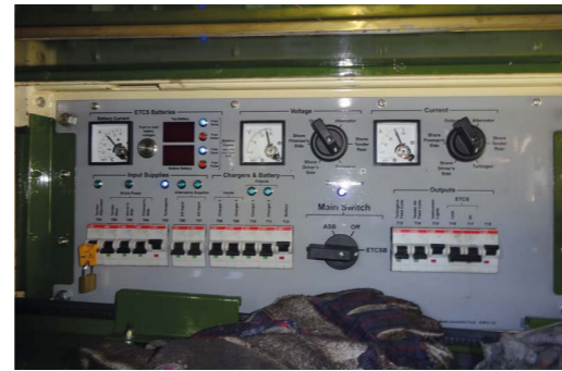
New Meiningen T2 turbogen under test, providing over 30A, including power to Load Bank and batteries.
