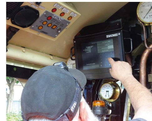
Arther Bull of Hitachi inputting data to the forward ETCS DMI prior to towed system testing.
