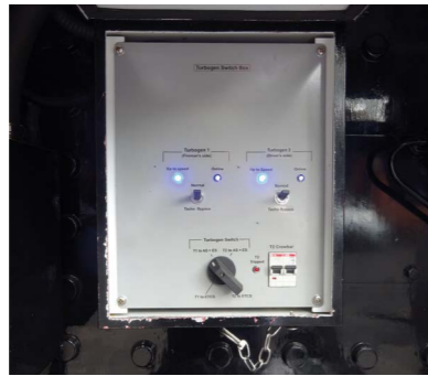
The new Turbogen Switch Box showing two turbogens operating together for the first time.
