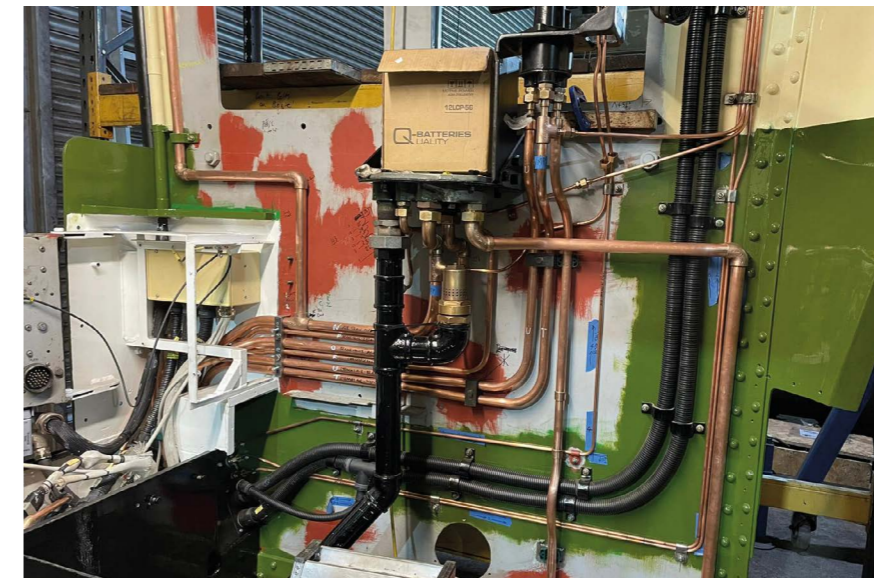
Some idea of the complexity of electrical conduit and air pipes in the cab can be gathered from this photo, taken before the overhaul was completed.
