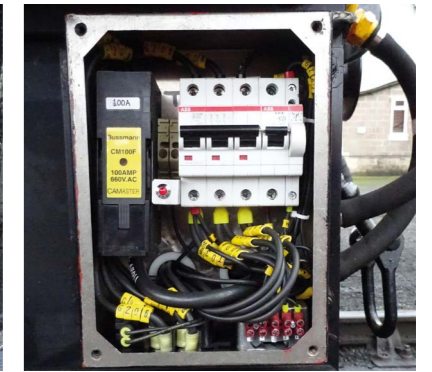
HCR relay (lower left) and tacho circuit (lower right) installed and ready for test.
