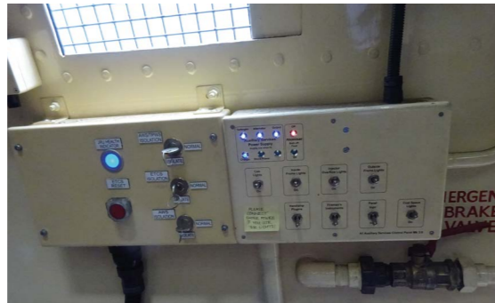
AS Control Panel showing turbogen and alternator both online and delivering power.
