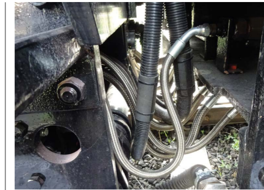
Engine-tender interface with all electrical, air, vacuum, water and steam connections in place.
